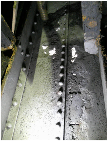
Extensive damage revealed at the tank bottom after blasting
