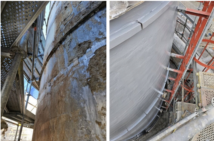
Tank walls damaged caused by corrosion Finished application
