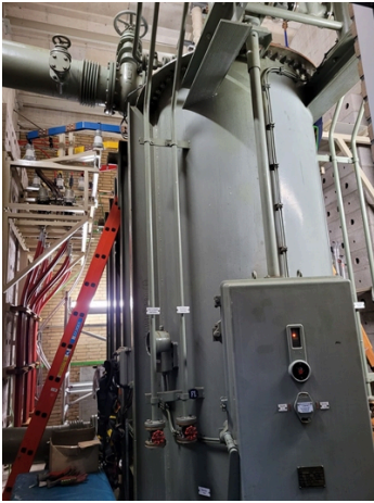
Transformer to be repaired.
