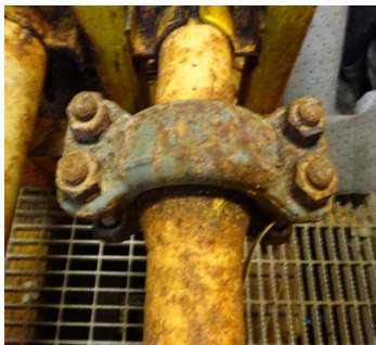
Corroded hub connector
