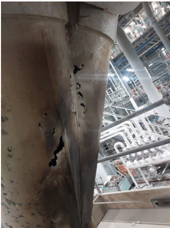
Ash chute had worn due to sliding abrasion
