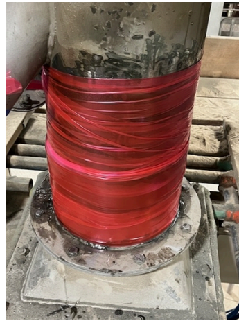
Belzona 1983 SuperWrap II is applied then Belzona 9382 release film is applied to consolidate application
