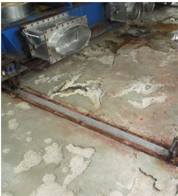
Floor damage caused by Succinic Acid
