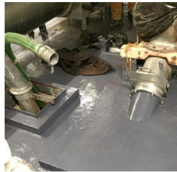
Second coat of Belzona 4311 around floor step up's and piping equipment through floor.
