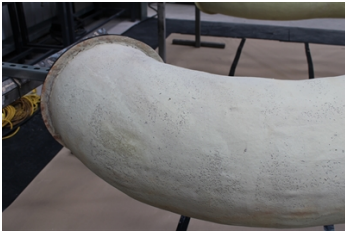
GRP Pipe Showing Crack
