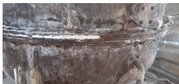
Condition of vessel circumferential flange
