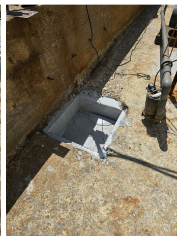
The sump after pouring a slurry mix of 4111 around the former. Application complete.
