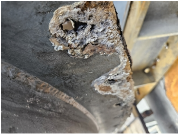
Flange with Sulfuric Acid Damage
