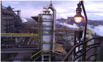
Overall view of the scrubber.
