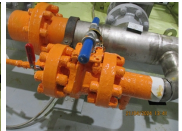
BELZONA 3412 CAN BE APPLIED TO ALL GEOMETRIES AND SEAL THE FLANGE AND FASTENINGS, EASY INSPECTION AND RESEAL.
