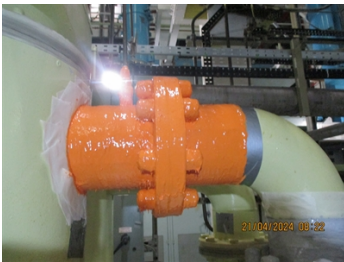
FLANGE & FASTENINGS PROTECTION
