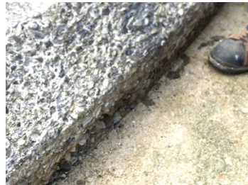
Damage after it was cleaned.
