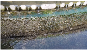
Constant water running over the weirs has caused damage to the concrete
