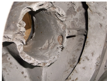
Up close view of the damage.
