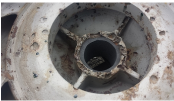
Original condition after opening the pump.
