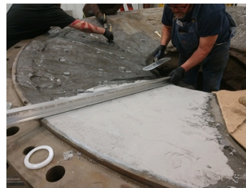
Applying Belzona 4911 Conditioner in the background, and applying Belzona 4111 using a guide to achieve the proper profile.
