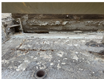
Worn out seams on basins
