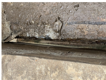
Current Gaps and Damage to Basin Seams
