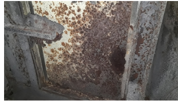
A close up of the general condition of the internal bay's steelwork
