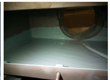
Both the bottom and the walls were treated with the product Belzona 1593.
