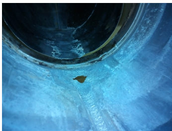
Damaged bottom and walls of the boiler.
