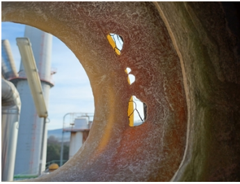
Severe damage to glass fiber necks and flanges
