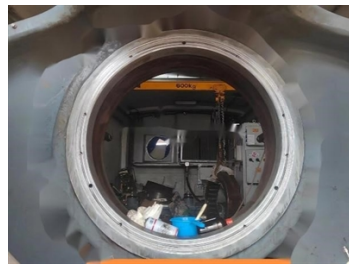
Sealing face before repair
