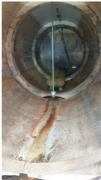
Damaged tank bottom
