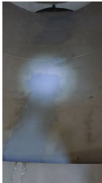
Fixed tank bottom
