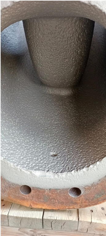
Pitting damage appeared after blasting
