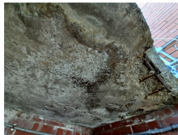
Stairwells showing severe spalling with possibility of falling concrete
