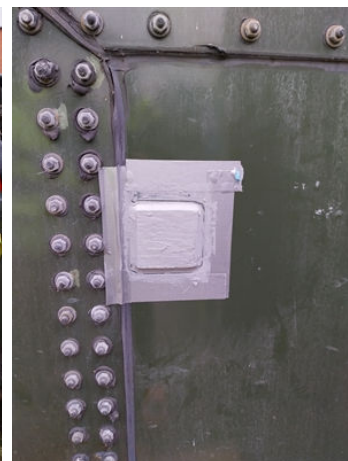
The solution ensures that no further corrosion can spread and weaken integrity of tank
