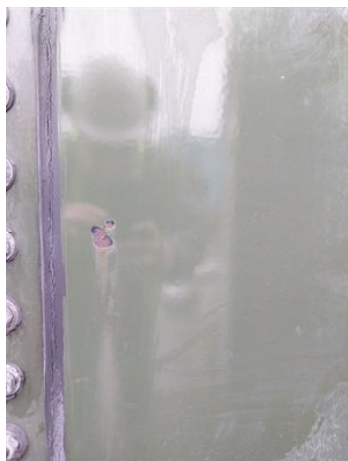
Several areas of external corrosion/damage were identified
