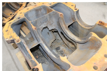
Severely eroded pumps with multiple through wall defects
