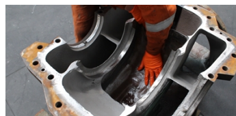
Through wall defects and missing metal is rebuilt
